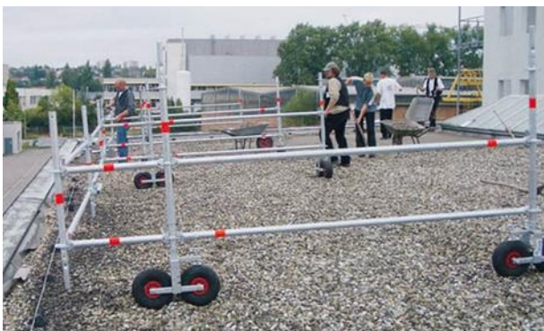
Figure 2 - Example of temporary railings.
