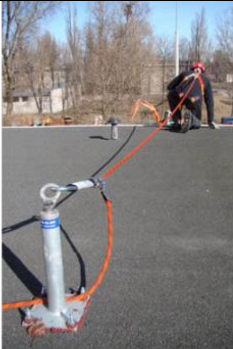
Figure 1 - Fixed anchor point with a rope that is long enough to prevent the employee from reaching the place where he is exposed to the fall hazard.
